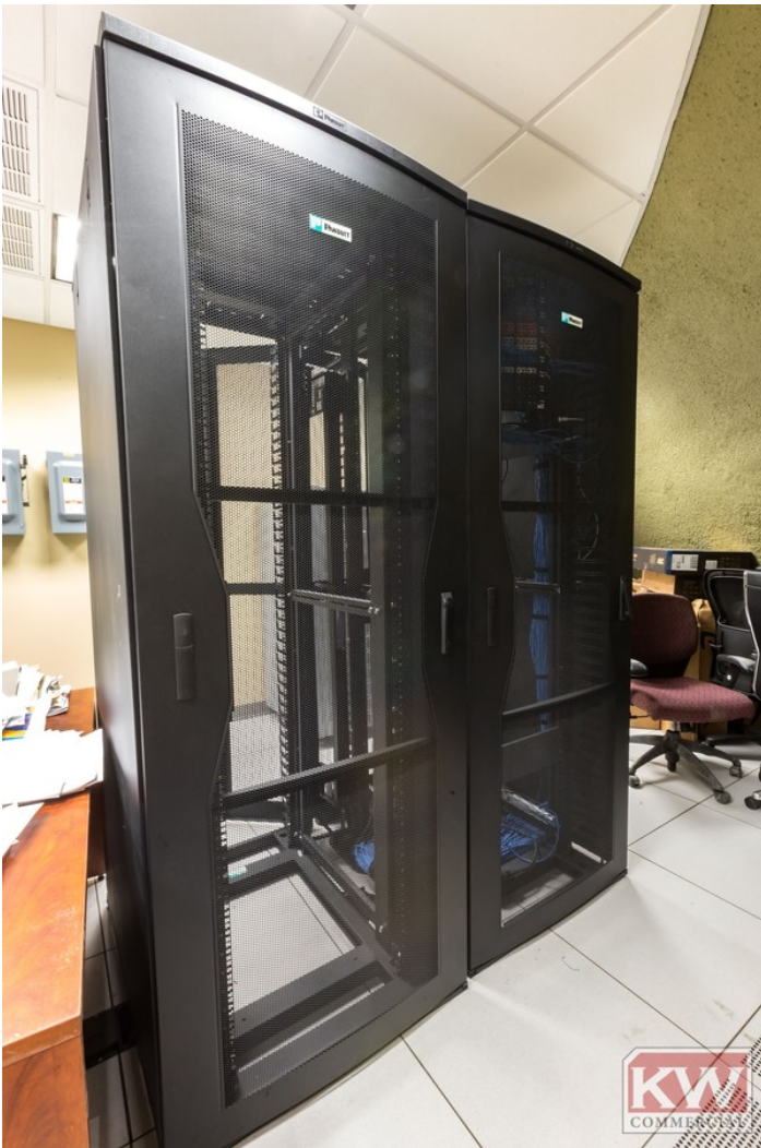
Dome B - Data storage
