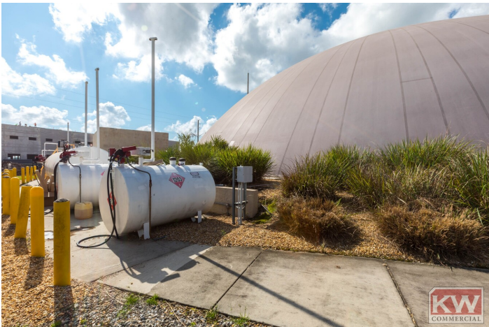
On site fuel storage
